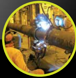
ENDEAVOUR ROCHELLE - UK TECHNIP – Evanton Spoolbase
